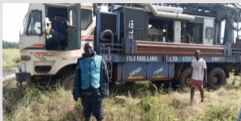
NaCSA GPC III PROJECT EMBARKS ON BOREHOLES CONSTRUCTION IN KAMBIA, KOINADUGU AND KONO DISTRICTS
