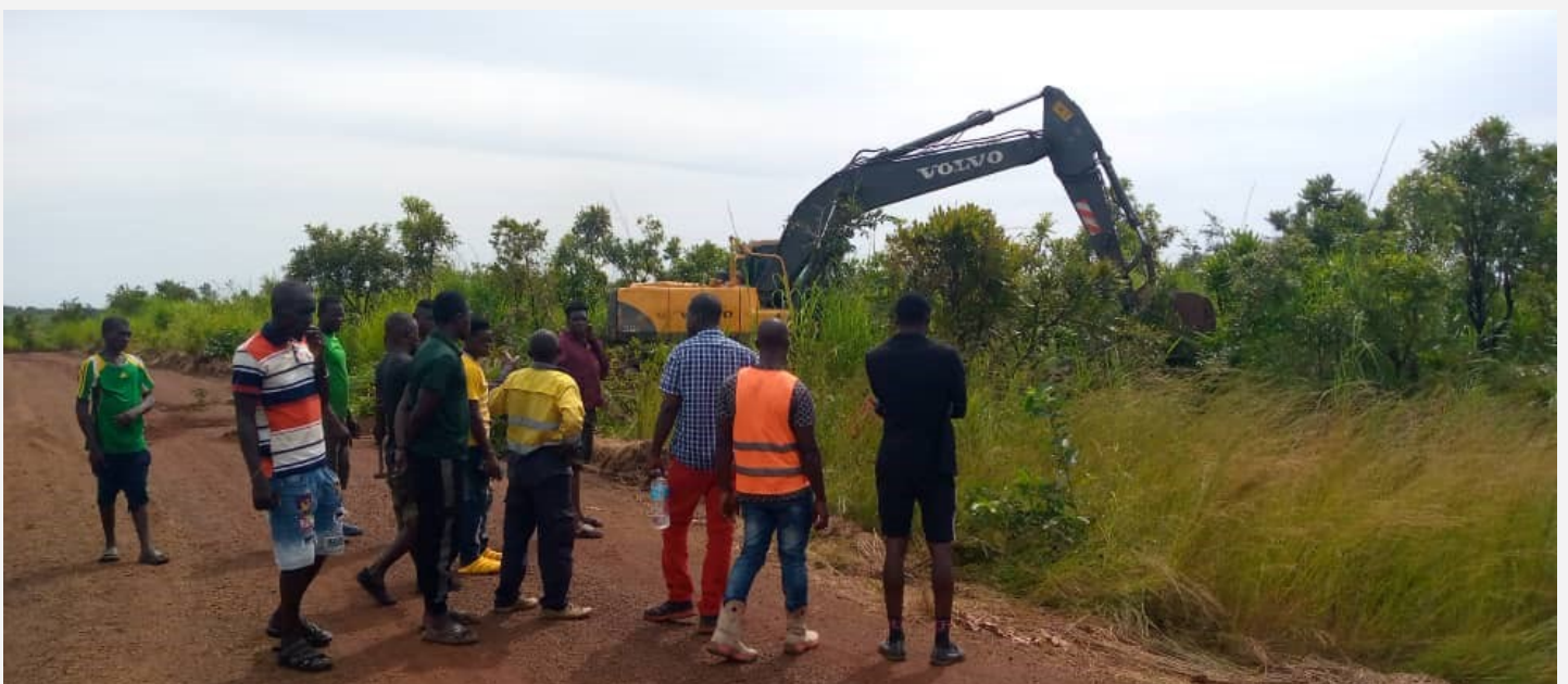
Assembling of equipment for the construction of Kumrabia to Mabang, and Matuku 2 to Mafolatha
