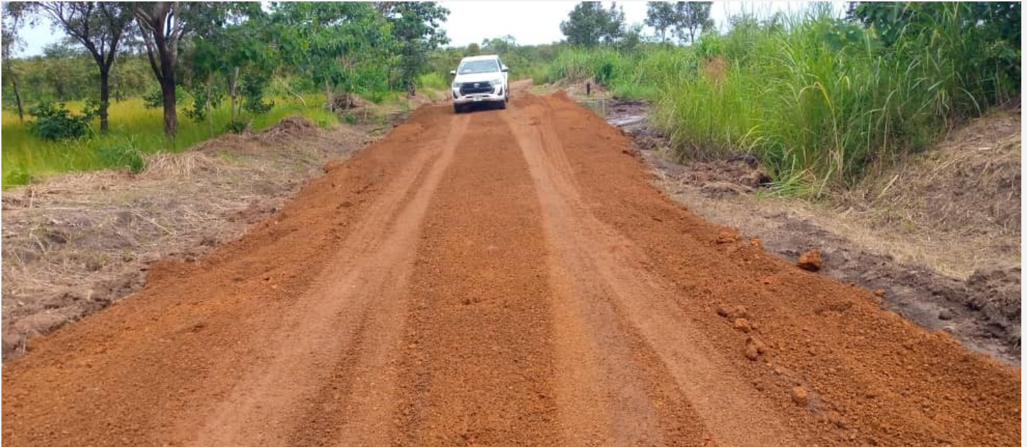
Kumrabia to Mabang, and Matuku 2 to Mafolatha under rehabilitation by the SLCDD II
